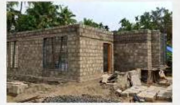
Masonry work of ground floor is finished. Preparing for casting floor slab.
