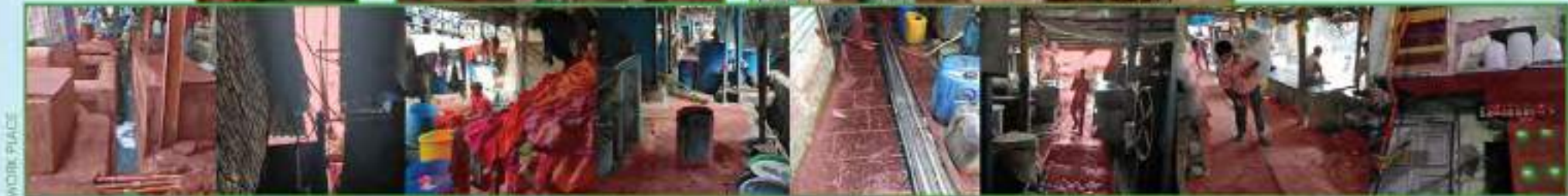
Open drainages throughout site causing pollution and accidental fall. Openings to sky is too narrow and small, that water takes more time to get evaporated making surfaces slippery. Dhobighat as it been designed in 1990s lack the space to store large amount of clothes during the washing. Circulation spaces is interecepted by washing machines, indicating the spatial constrain dhobighat is facing. Exposed water intake pipes going through circulation spaces. Lack of natural light in circulation spaces. Circulation spaces defined by temporary elements in most parts lack proper pavement. The main switch board near dwelling without proper safety.
