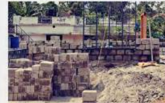
Window frames being installed in site simultaneously with masonry for strong bonding
