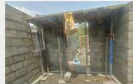
Shuttering process done for lintel beam, extending lintel beam to make storage spaces in kitchen.
