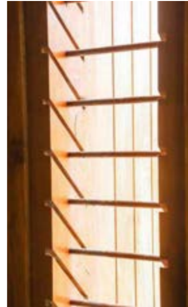
Louvered vents Grooves for louvered frost glass vents in the restroom slit windows with MS safety rods
