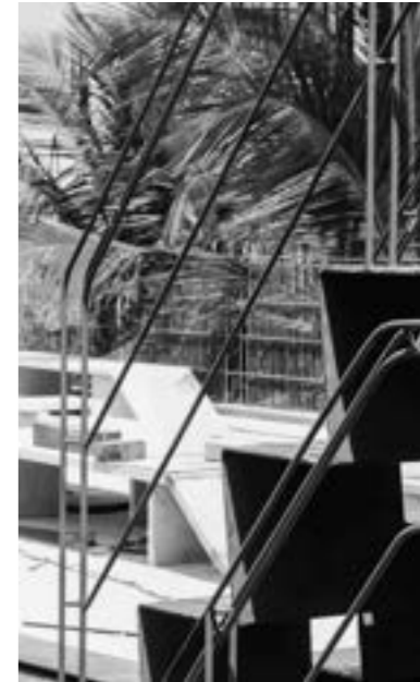
Folded metal plate stair MS plate folded to form a single flight, parallelly another flight is staggered for left-right step access to make a single user stair to terrace.
