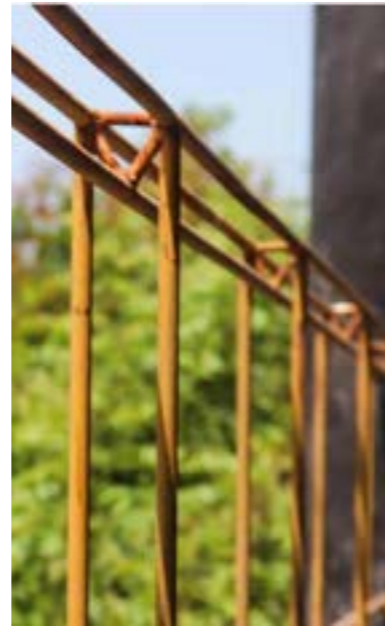
Three dimensional mesh rail The triangulation drops down to the floor for vertical support
