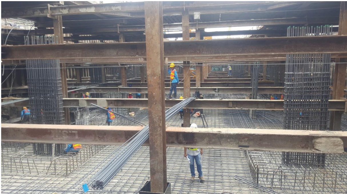
Pic 2 RC. Flat Slab for underground floor and Post-Tensioned slab for typical floor.
