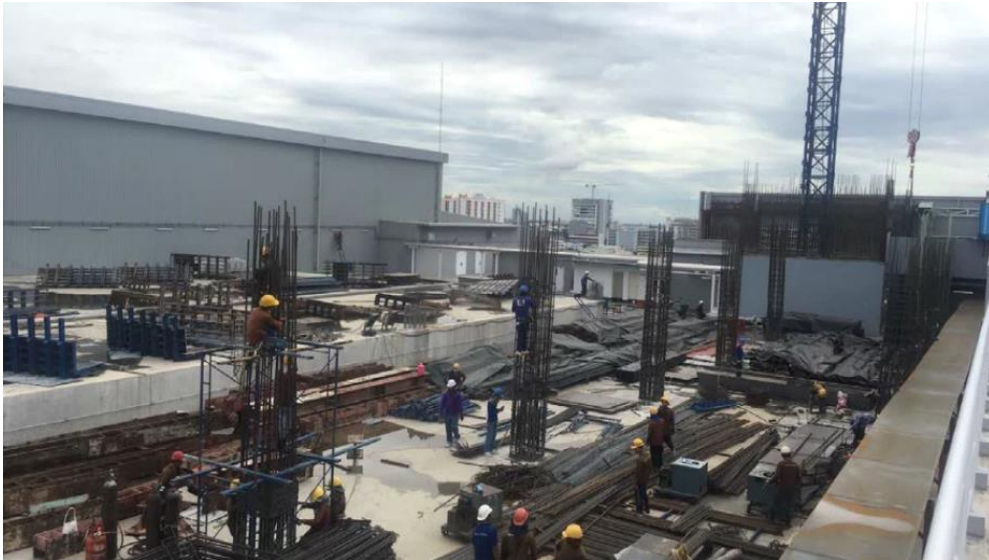
Pic 1 Prepare site of work above retail area on 5 th floor for construction hotel tower.
