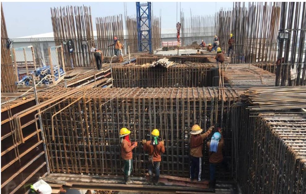
Pic 2 RC. Transfer Beam to change span of column for hotel tower.
