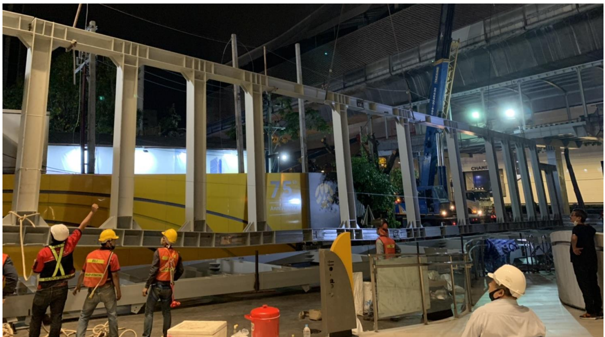
Pic 2 Prepare Steel Vierendeel Truss for 30 m. long span bridge on site.
