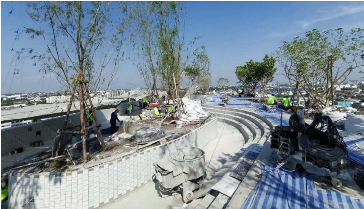
Pic 4 RC. Flat Slab with Band Beam for landscape and swimming pool on 15 th Floor.
