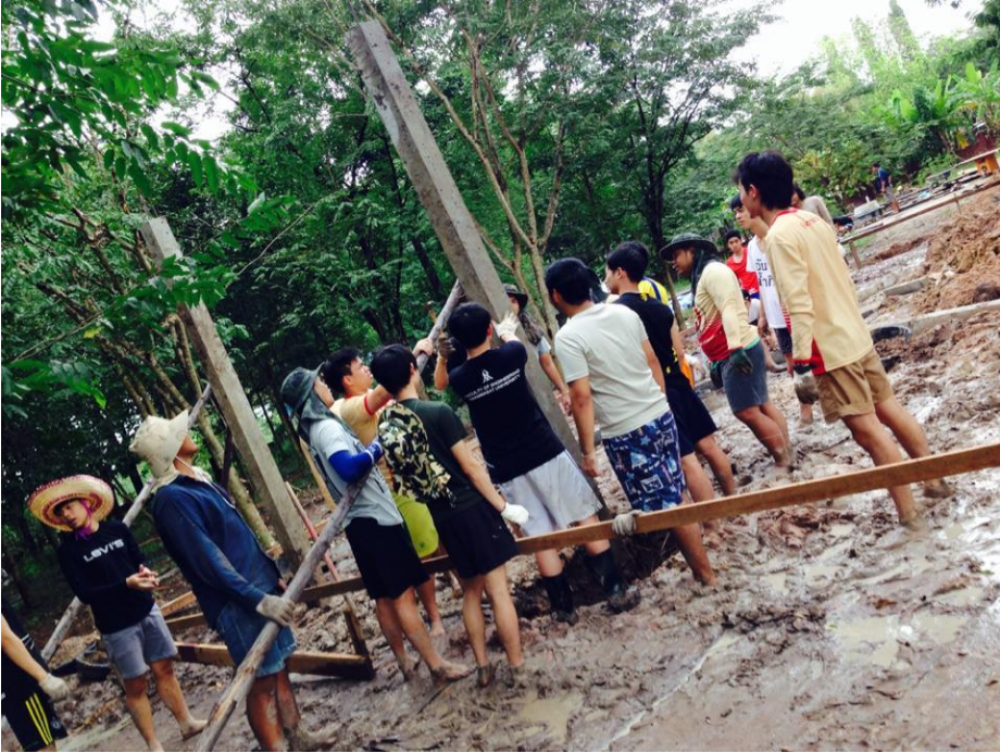
Civil engineering camp activity for built school building at Bankaboktia School, Chachoengsao.
