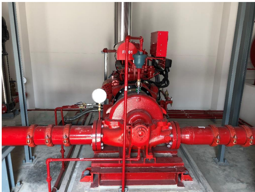
FIG.8 Horizontal split case fire pump at Yellow Wood 6 New Warehouse
