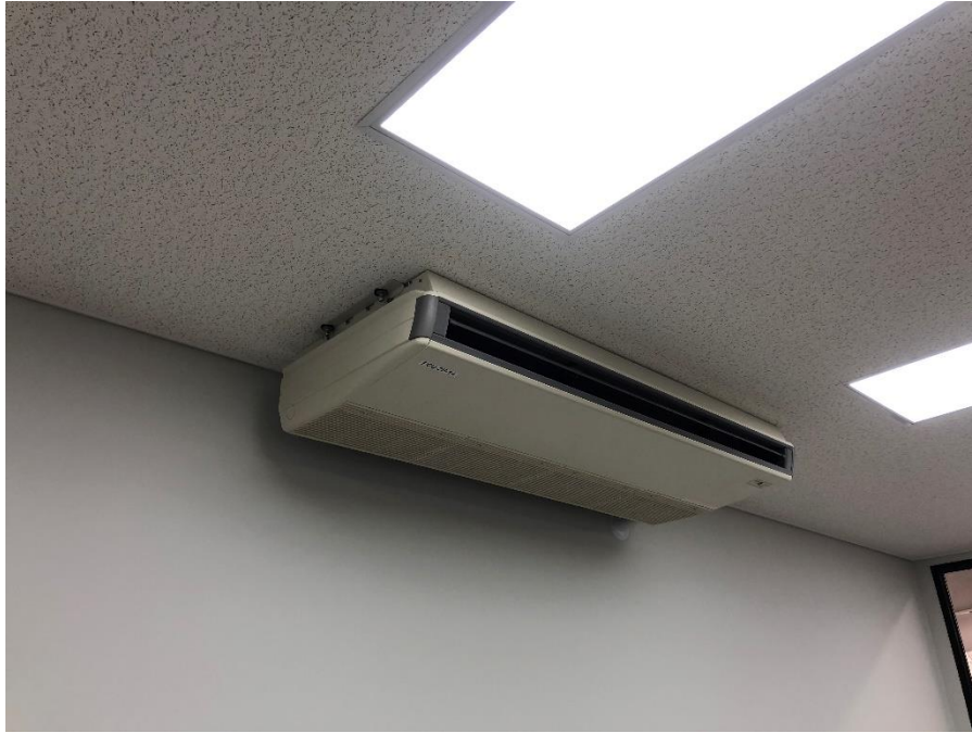
FIG.13 Office area (Air condition space) at ASRB New Factory
