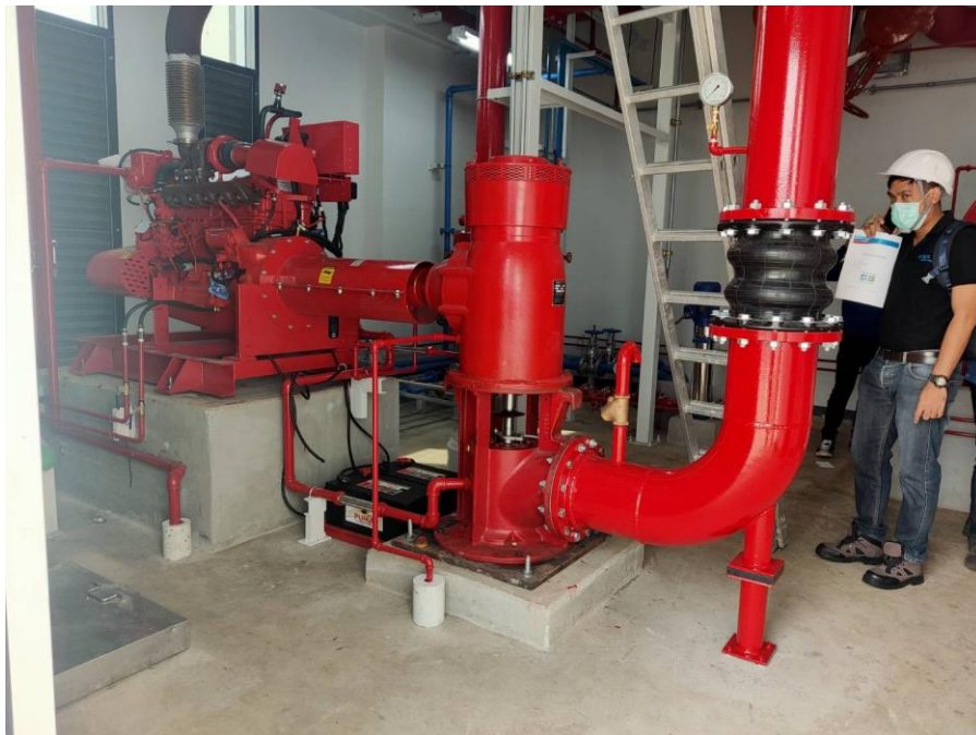
FIG.16 Vertical turbine fire pump at Amata Summit Warehouse & Distribution Center
