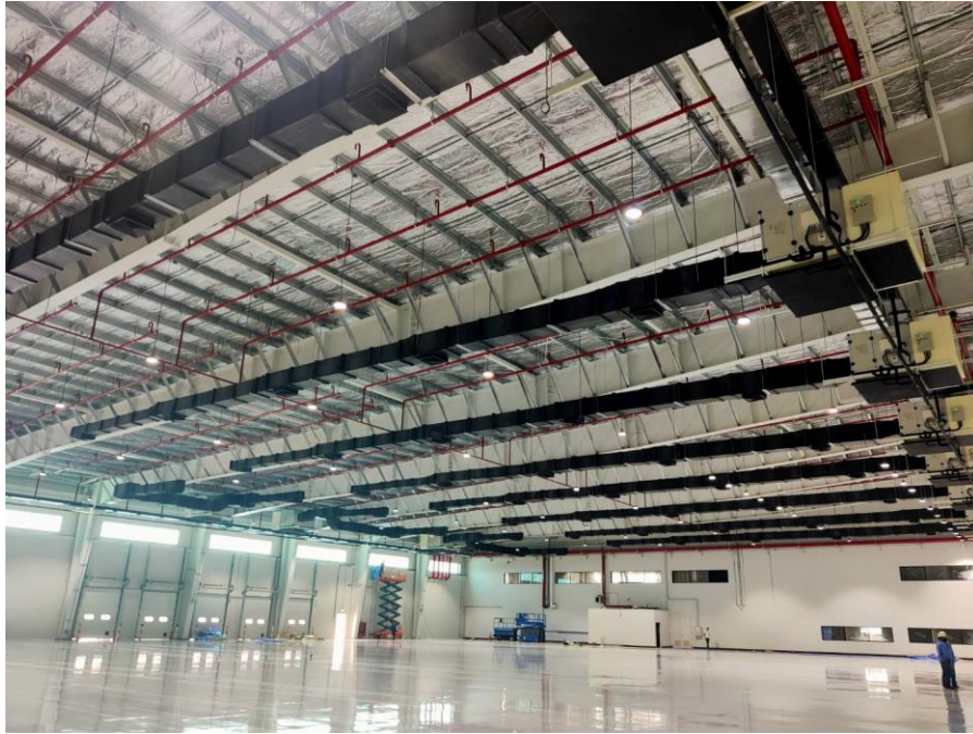
FIG.17 Warehouse area (Air condition space) at Amata Summit Warehouse & Distribution Center 1
