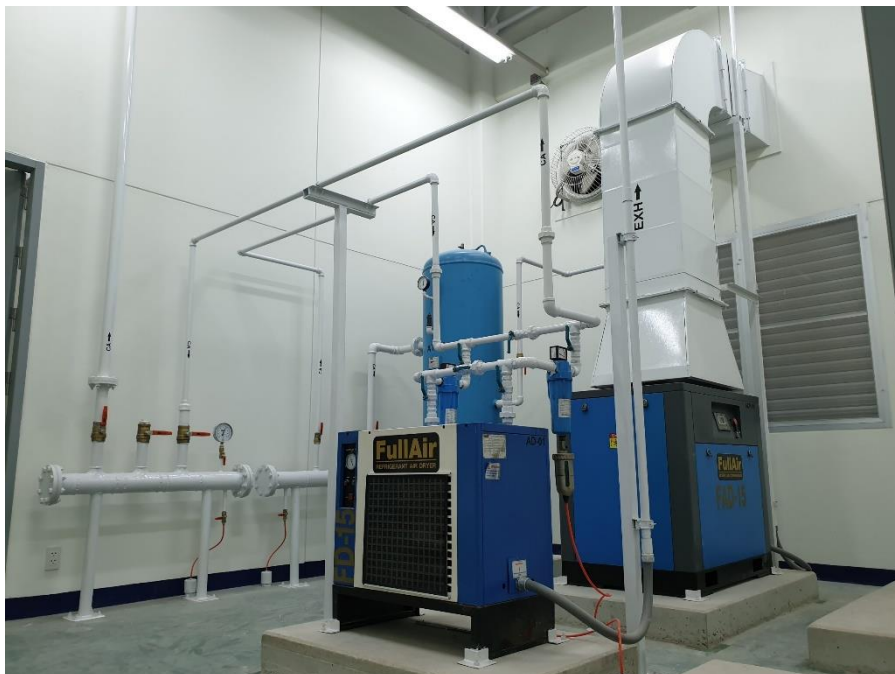
FIG.2 Air compressor room (Main equipment by owner) at Siam Mizusho New Factory
